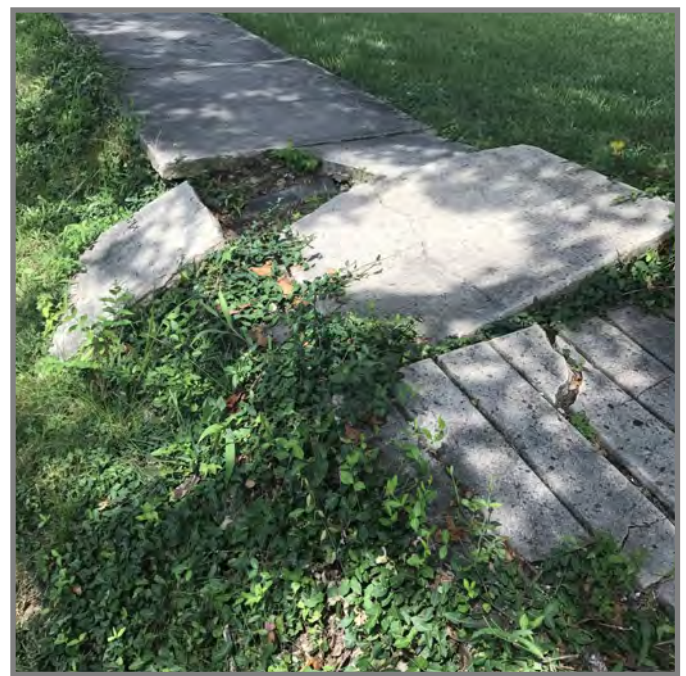
An example of sidewalk deterioration in Old Town.
