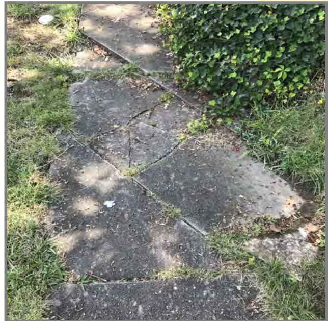
Shown above are two sidewalk segments on James Boulevard in Old Town. One segment is in relatively good condition; the other is in need of repair.
